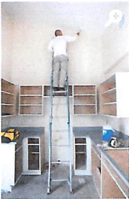
Alberto Castillo paints inside one of the houses in the Hatcher's Preserve development being built by Rural Neighborhoods in Immokalee, FL on Tuesday, May 17, 2016. (Photo by Gregg Pachkowski/Special to the Daily News)
